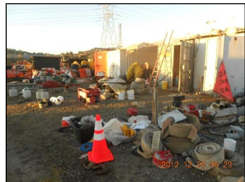
Stored materials should be organized and placed within containment areas when not in use.
